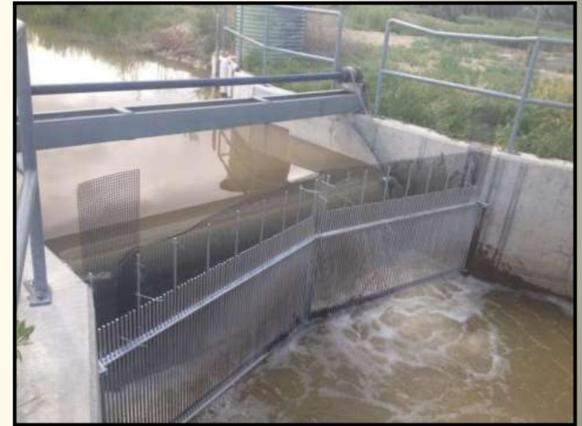
Picket weir at inlet gate
