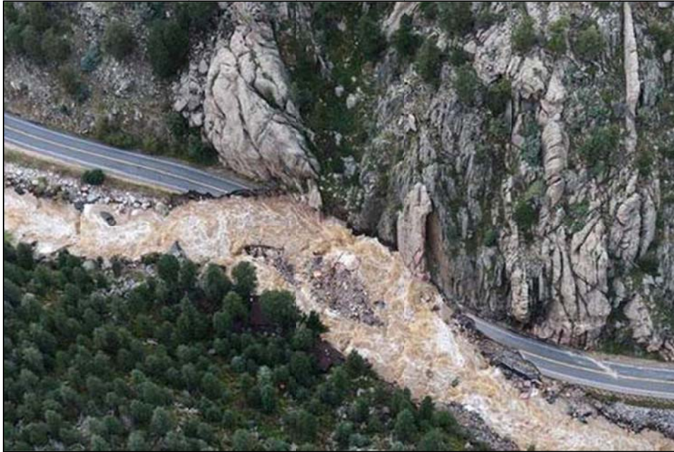
Figure 14. September 2013 Flooding, Highway 34 Big Thompson Canyon, Highway Damage (Photo by Andy Cross, The Denver Post)
