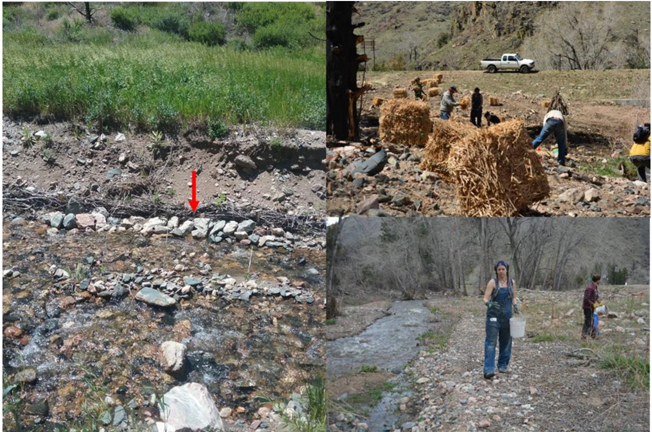
Figure 9. Red arrow indicating a willow fascine installed along the bank in Skin Gulch (left). Volunteers laying mulch over newly planted & seeded floodplain area in Skin Gulch (upper right). Volunteers seeding the floodplain at Skin Gulch (Lower left).
