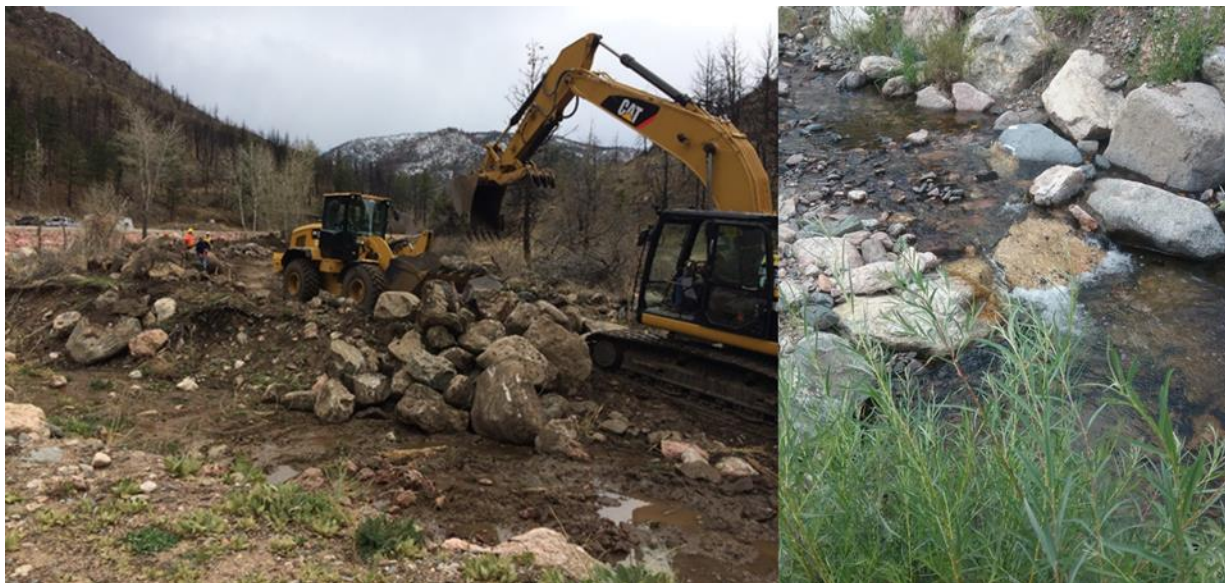
Figure 8. Heavy equipment working to create stable channel formation at Skin Gulch, 2015 (Left). An example of a rock/log grade control structure installed with heavy equipment at Skin Gulch (Right).
