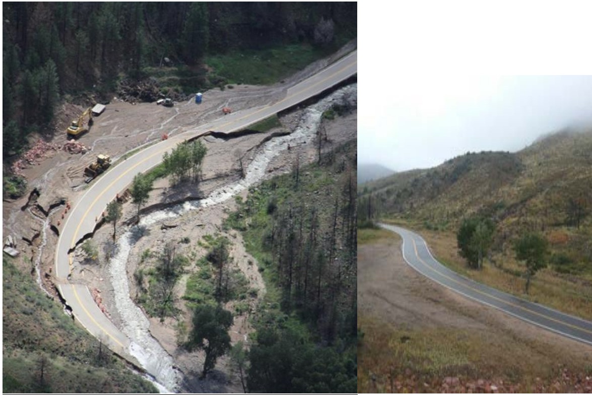
Figure 7. (Left) Skin Gulch showing damage resulting from rain event after the High Park Fire. Image shows the damage to Stove Prairie Rd and Co-14 and excessive sediment being delivered to the Poudre. Photo courtesy City of Ft Collins. (Right) Stove Prairie Road
