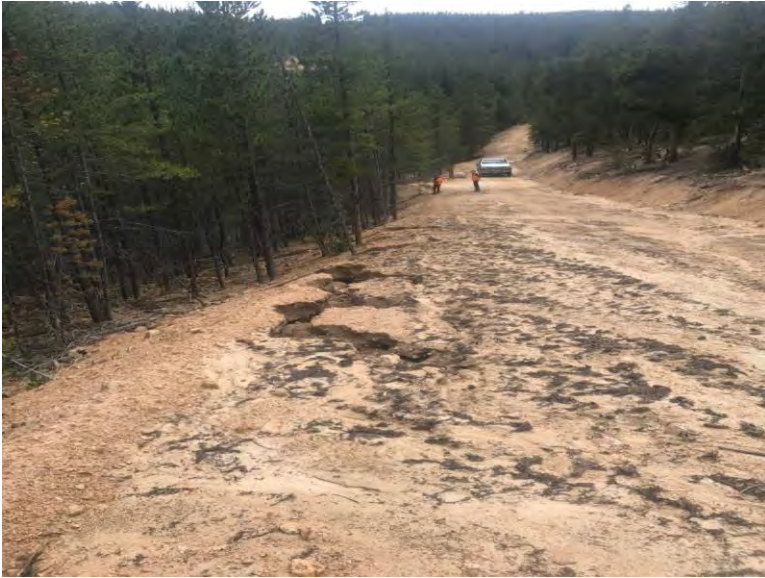
Road Damage above Little Frying Pan on Powerline Road
