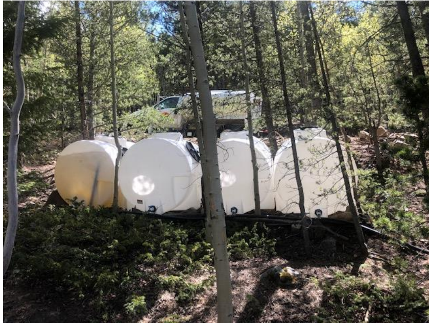
Figure 14 - Manifold System with Four 500-gallon Tanks
