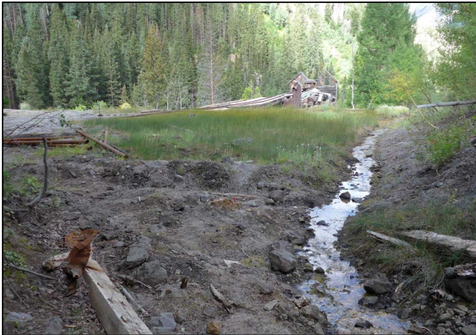
Figure 8. A. Adit discharge flowing onto, over and through the waste rock pile at the Michael Breen Mine before implementation in 2014. The top of the load out structure is in the background. B. The diversion ditch was constructed in fall 2014 and routes the adit discharge around the waste rock and the load out.
