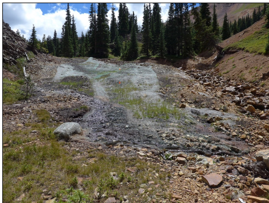
Figure 5. A. Waste rock pile in Gray Copper Gulch at the Vernon Mine site in 2014. The 1,500 cubic yards of waste was excavated in 2015 and placed in a repository away from the gulch (upstream view). B. The excavated area (upstream view) was amended with woody compost, seeded with high elevation herbaceous species, and covered with aspen blankets in 2015. This photo was taken in 2017, two years after seeding.
