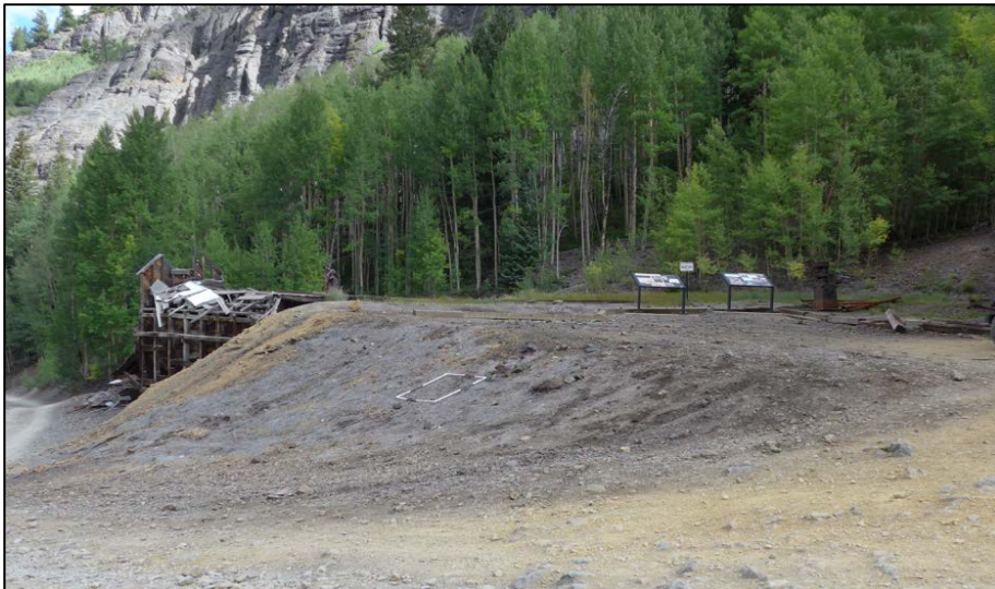
Figure 7. A. Michael Breen Mine site before implementation in 2014. The adit discharge flowed over and seeped through the waste rock pile and loadout structure before crossing the county road and draining into the Uncompahgre River below. B. A diversion ditch was constructed in fall 2014 to route the adit discharge around the waste rock and into an existing drainage behind the load out structure. The waste rock was amended with biochar, seeded with a high elevation herbaceous seed mix and covered with aspen mulch shown in this photo. C. Photo-point of waste rock pile in 2017 showing that very little vegetation established after treatments in 2015 (photo B.)
