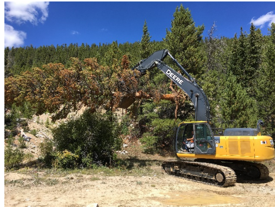
Figure 6.3: Photo showing excavator transporting root wad from Silver Spoon to Streamside area.
