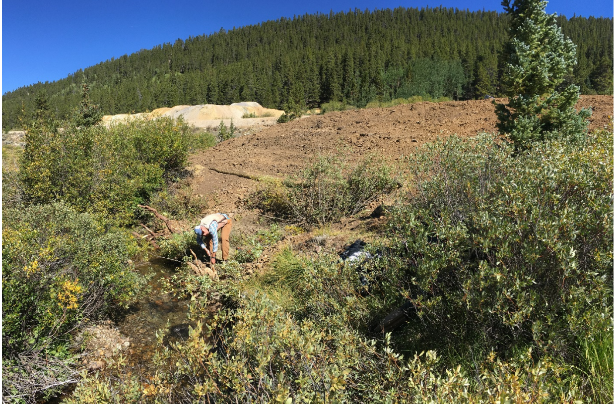
Figure 6.4: After conditions showing graded and amended pile with establishment of clean floodplain bench. A total of three root wads were installed in the bank in conjunction with 12 whole willow transplants and six sedge mats to provide bank stability and trout habitat. TU staff is shown in the photo installing live willow cuttings into the bank.
