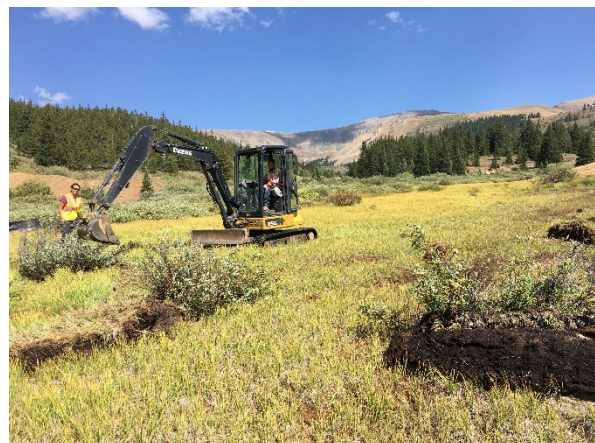
Figure 6.5: Mini-excavator shown installing whole willow clumps to the dead zone area downslope of the Valley Mine. Over 40 total willows were transplanted.
