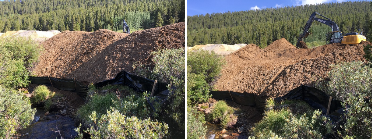
Figure 6.2: (Left) Before conditions showing Streamside tailings pile abutting Evans Gulch; (Right) During construction conditions with part of pile removed and graded as excavator benches its way down towards the bankfull elevation.
