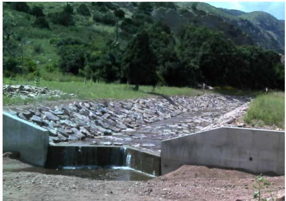
Riprap channel through Navigators
