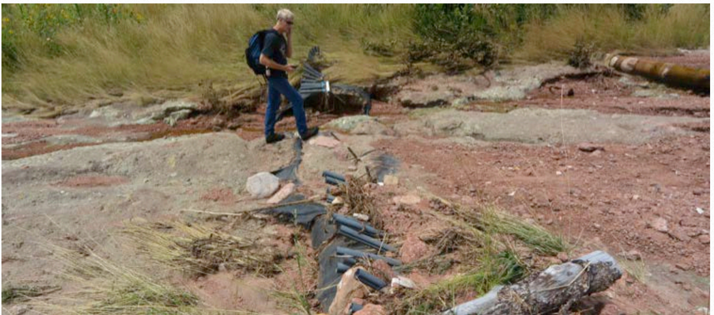
Damaged Whisker Sills: These were a new product recommended by a hydrologist, but they failed quickly.
