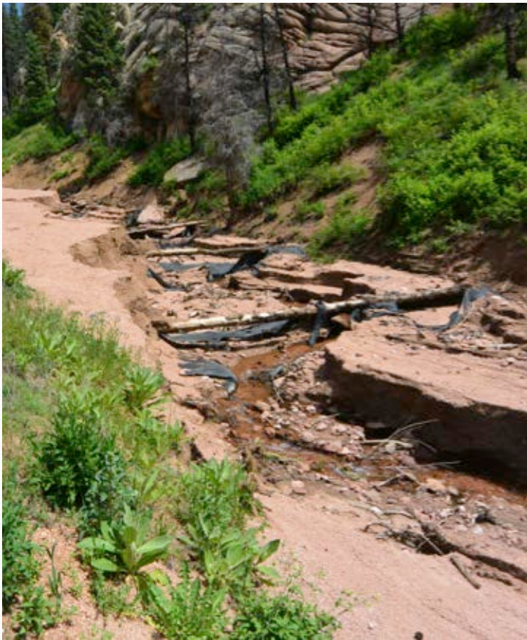
Failed sills in Middle Wellington
