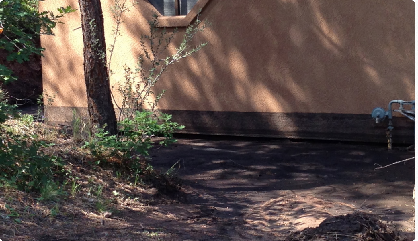
Mud flow line from a post-fire flood on a home in Cascade.
