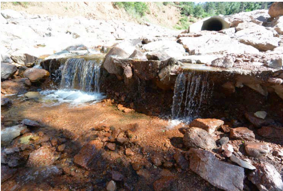
Grouted Rip Rap Channel functioning at risk as the toe begins to erode.
