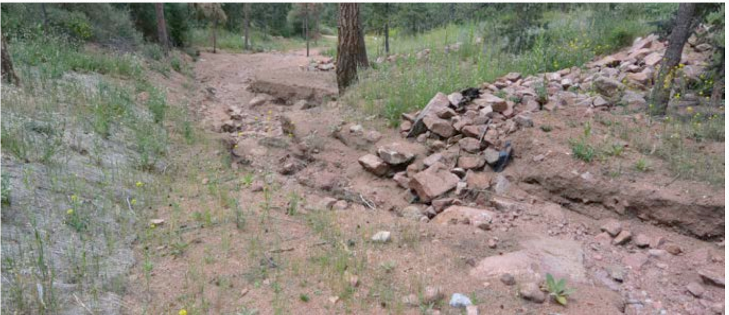
Bendway Weir causing channel down cutting in Lower Cascade Creek.
