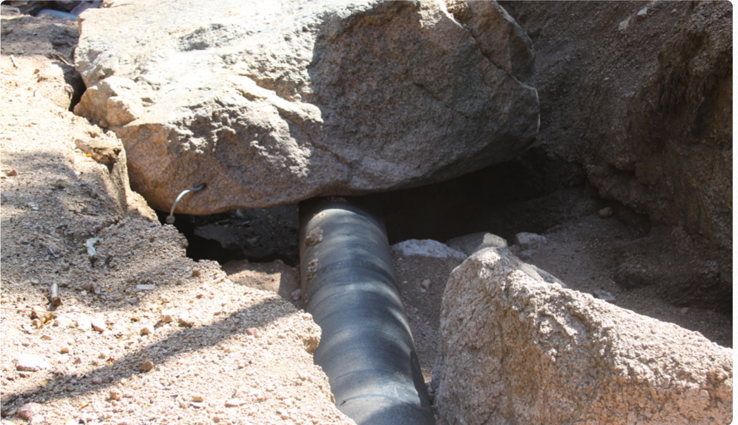
Post-fire flooding in 2012 exposed Colorado Springs Utility's backup pipeline from Rampart Reservoir, making it unsafe to run water through until repairs could be completed.
